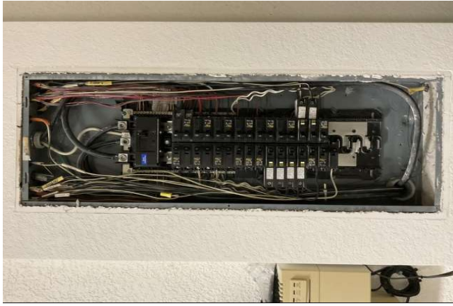
Inside Electrical Box
