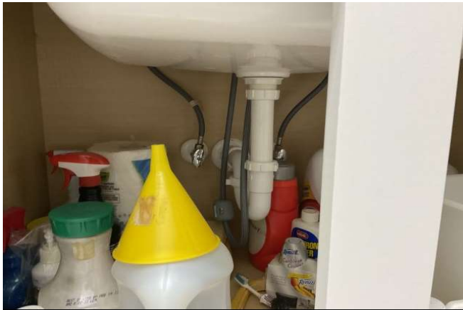
Plumbing - laundry sink
