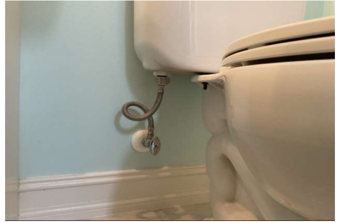
Plumbing - #2 bath toilet valve
