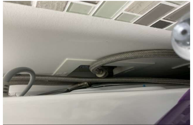
Washing Machine Outlet Box
