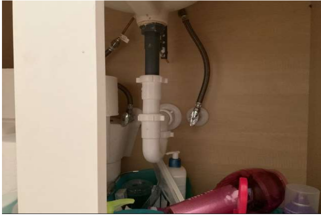
Plumbing - #2 bath sink
