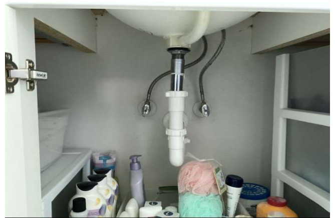
Plumbing - Master bath left sink
