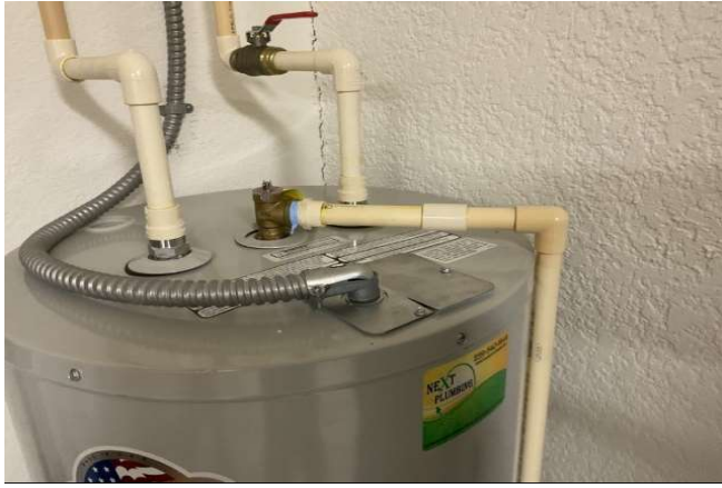
Water Heater T&P Valve
