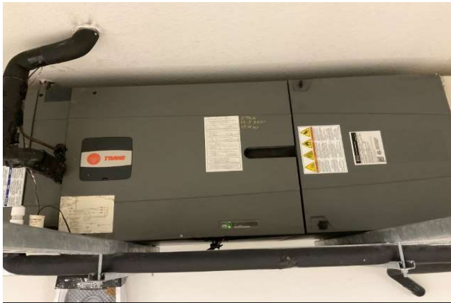
AC Air Handler
