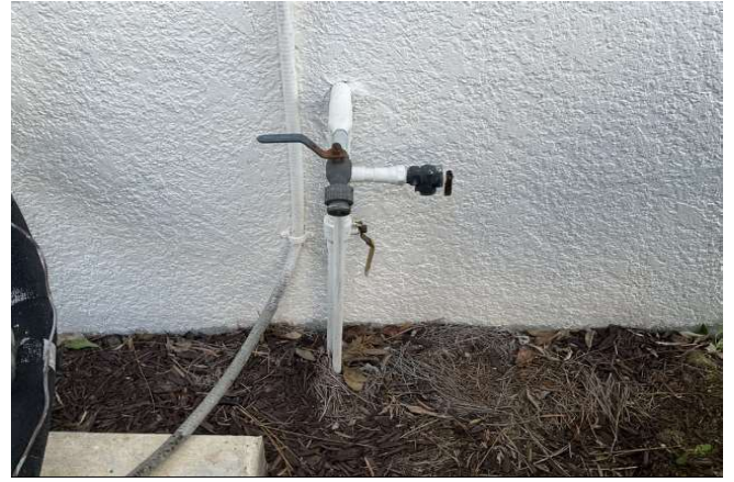
Water Main Shut Off
