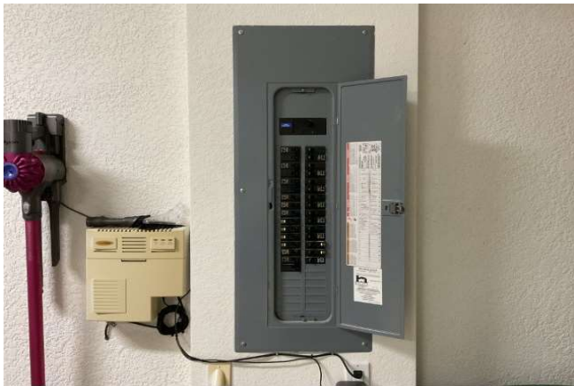
Outside Electrical Box
